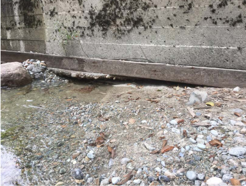
Left abutment scour, extends 700mm
