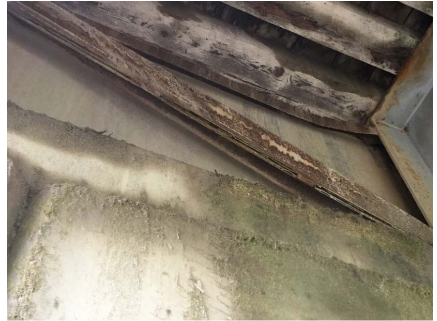
End bracing at right bearing heavily corroded
