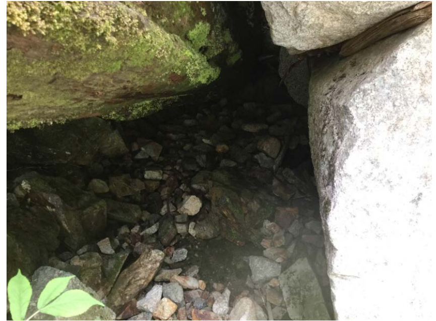
Scour noted behind upstream left abutment, extending up to 3m
