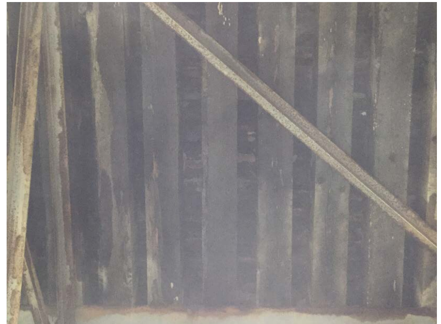
Indication of rot on subdeck
