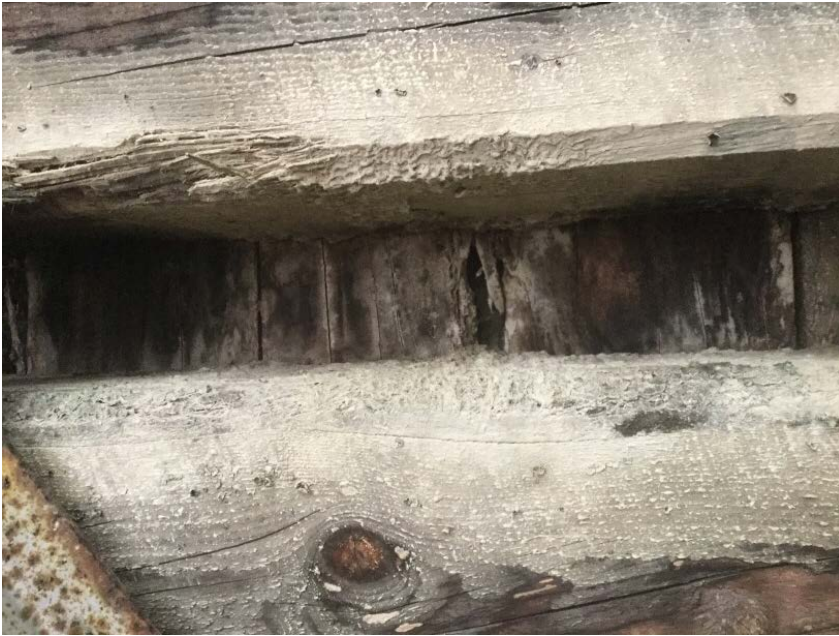
Tie and subdeck condition
