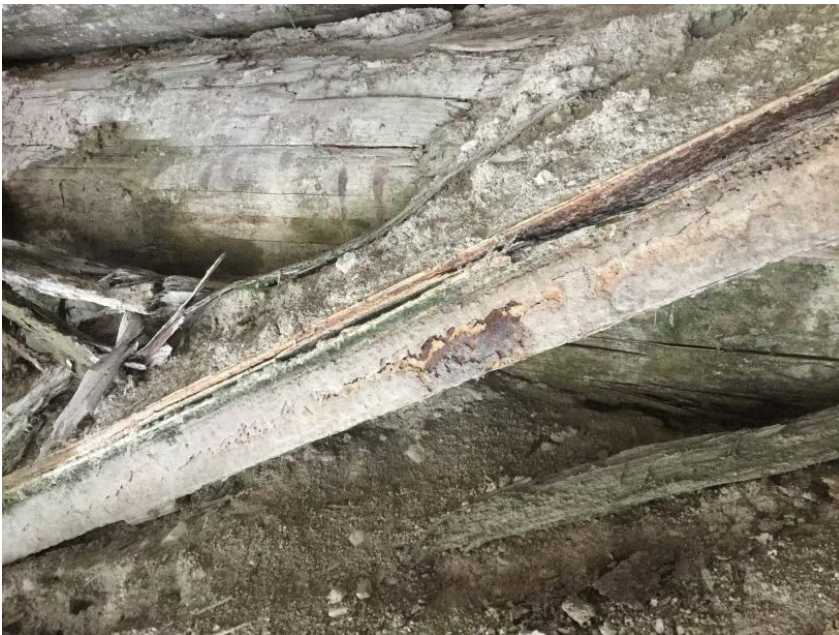
End bracing at left abutment heavily corroded
