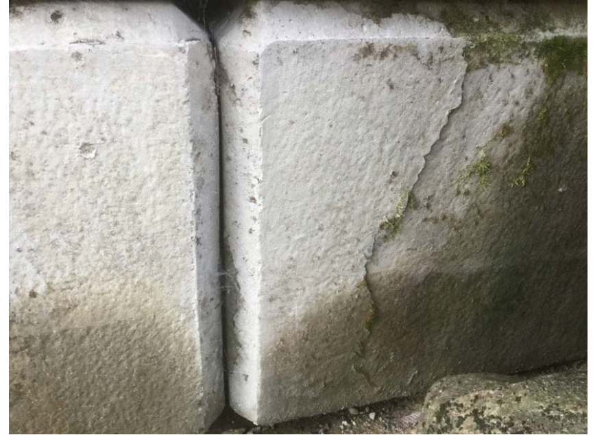
Bottom lock block at right abutment cracked
