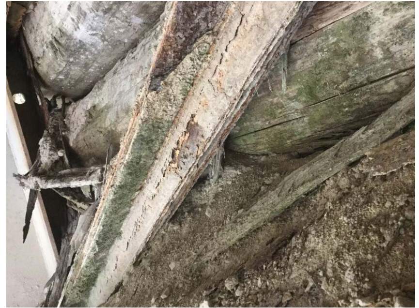
End bracing at left abutment heavily corroded
